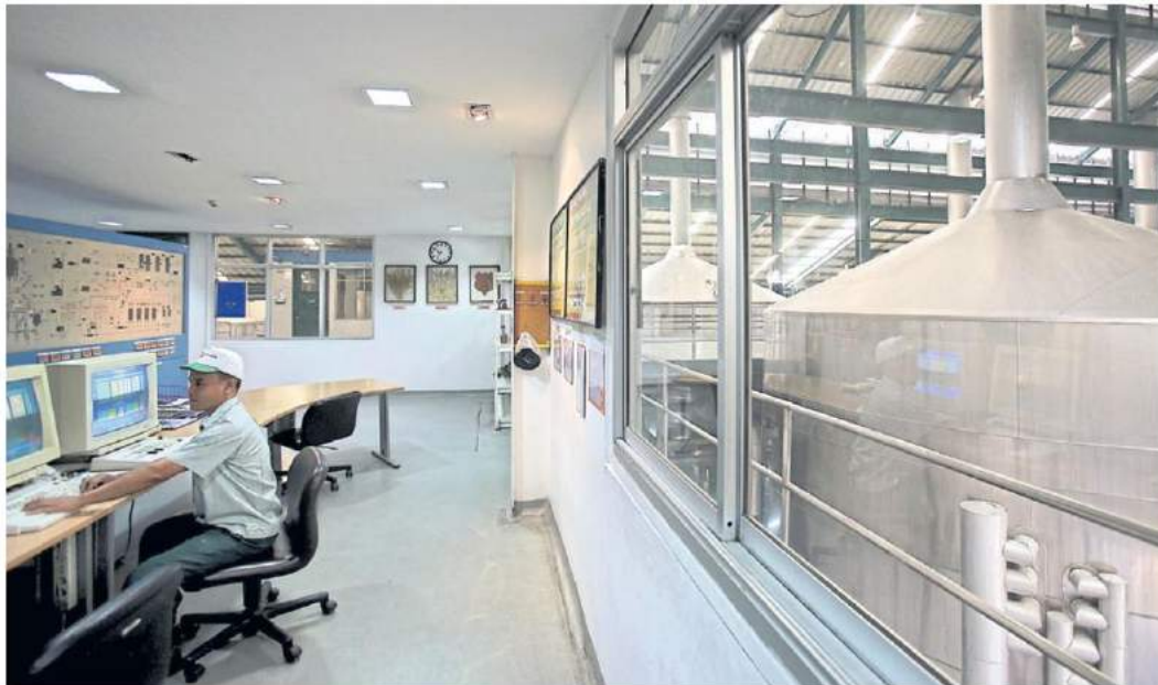
A worker sits in the control room of the water silo unit at Thai Beverage Plc's Beer Thip brewery in Bang Ban, Ayutthaya province.
